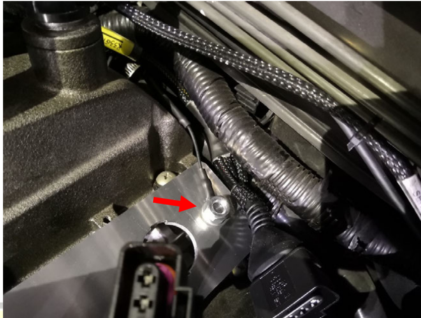
Figure 7 - Ground wire ring installed on the rear of the plate
